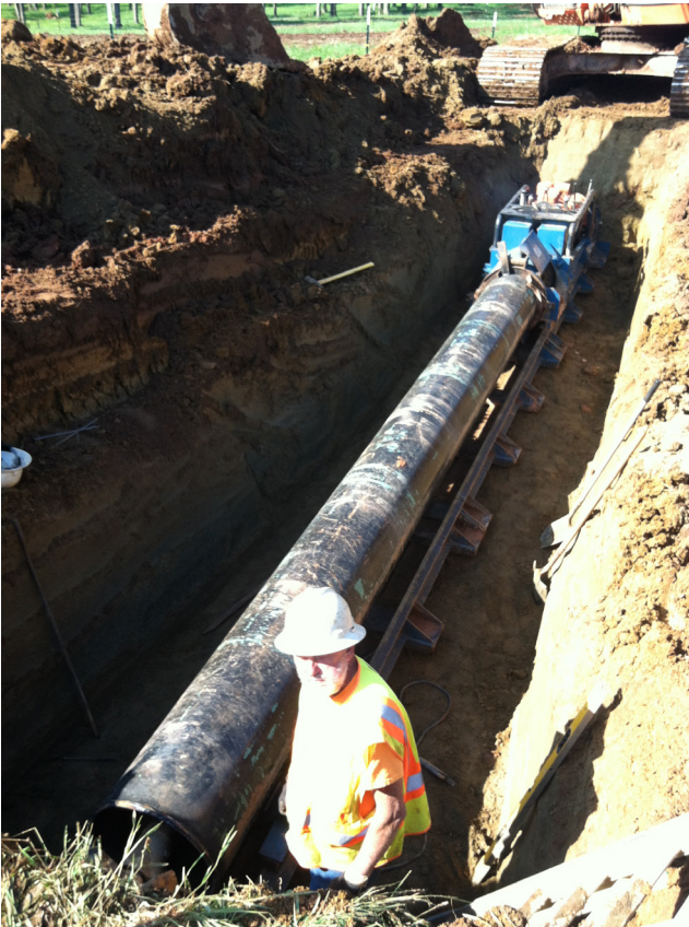
Some boring operations may be smaller to go under a large tree or driveway.
