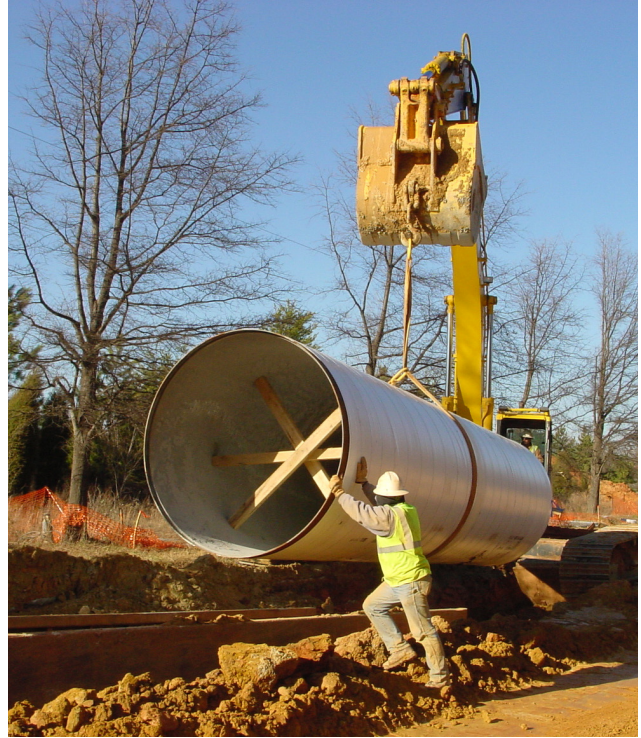
72-inch water transmission pipe to serve several neighborhoods.
