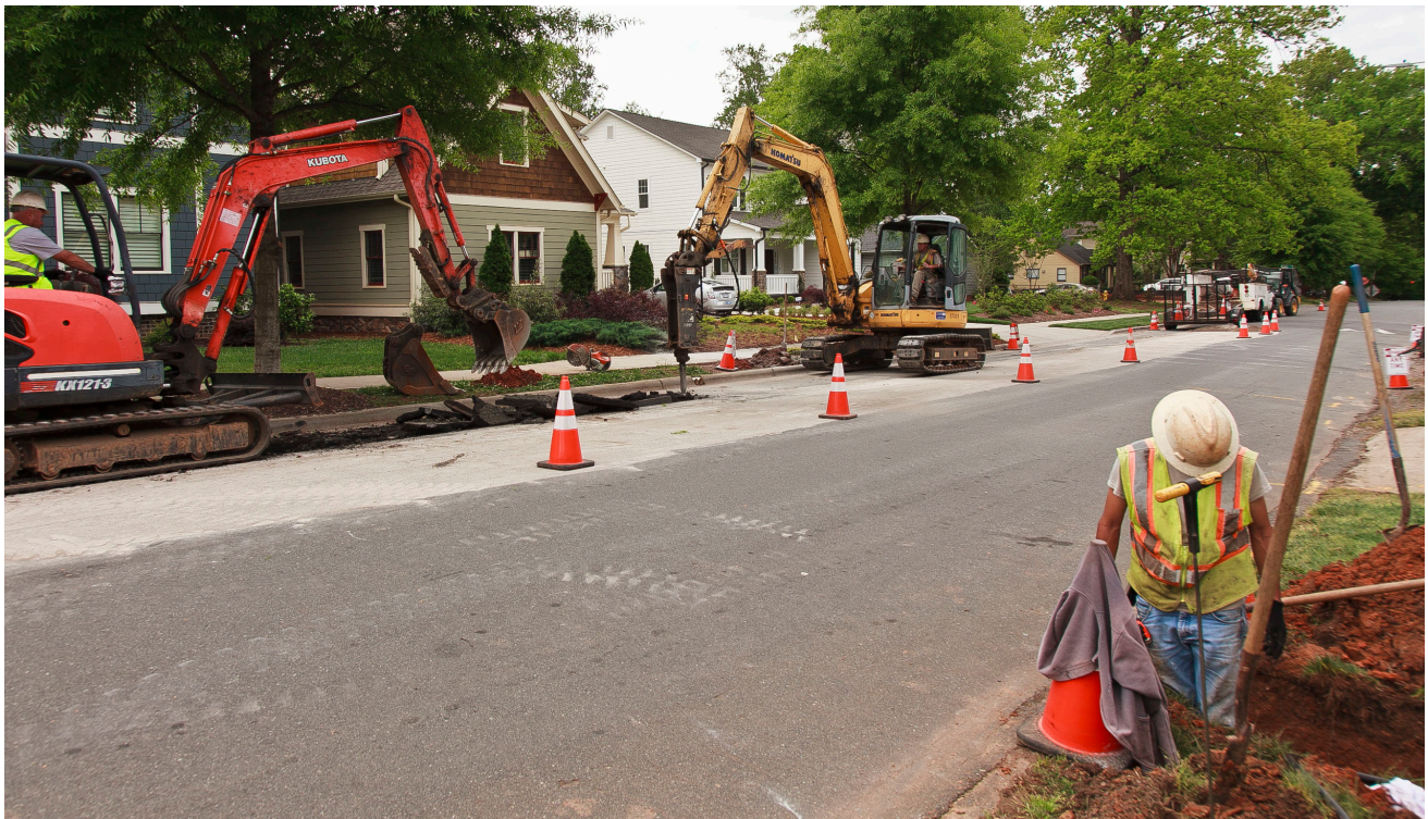
6-inch drinking water pipe replacement project including new service pipes to each water meter.
