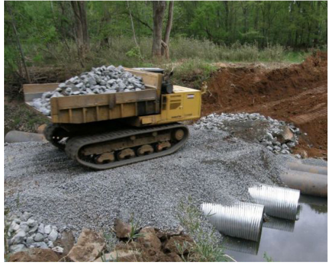
Contractors may create a safe creek crossing for equipment. Large pipes keep the creek flowing underneath.
