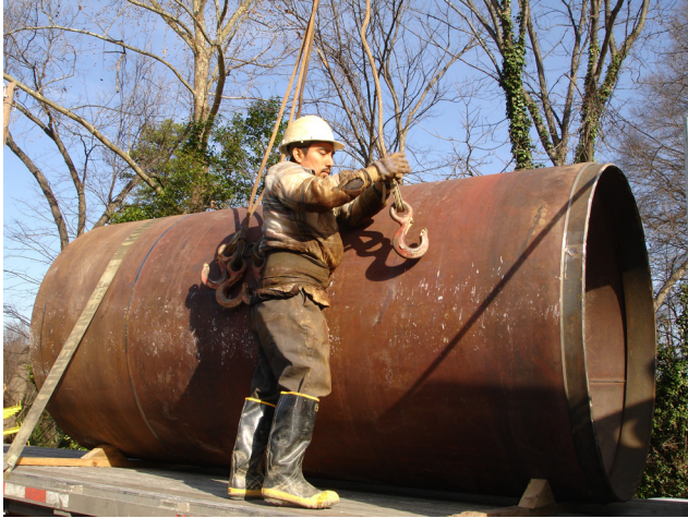
The pipe is installed inside a metal casing to protect the pipe, the street, and other infrastructure above the tunnel.
