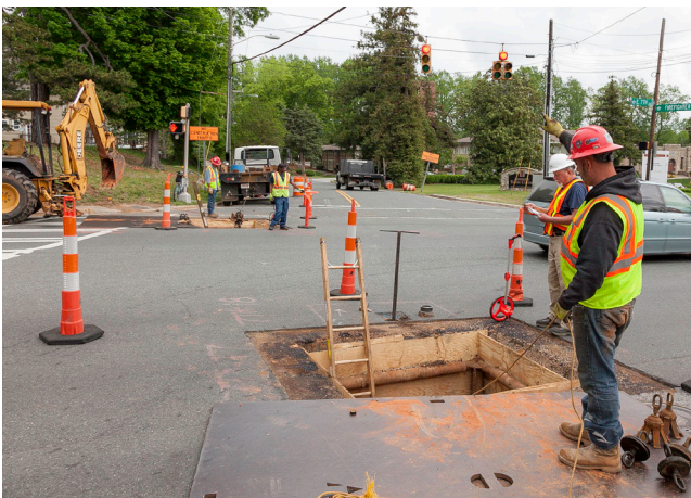
Crew cleaning underground pipe while customers are served with an above ground pipe.
