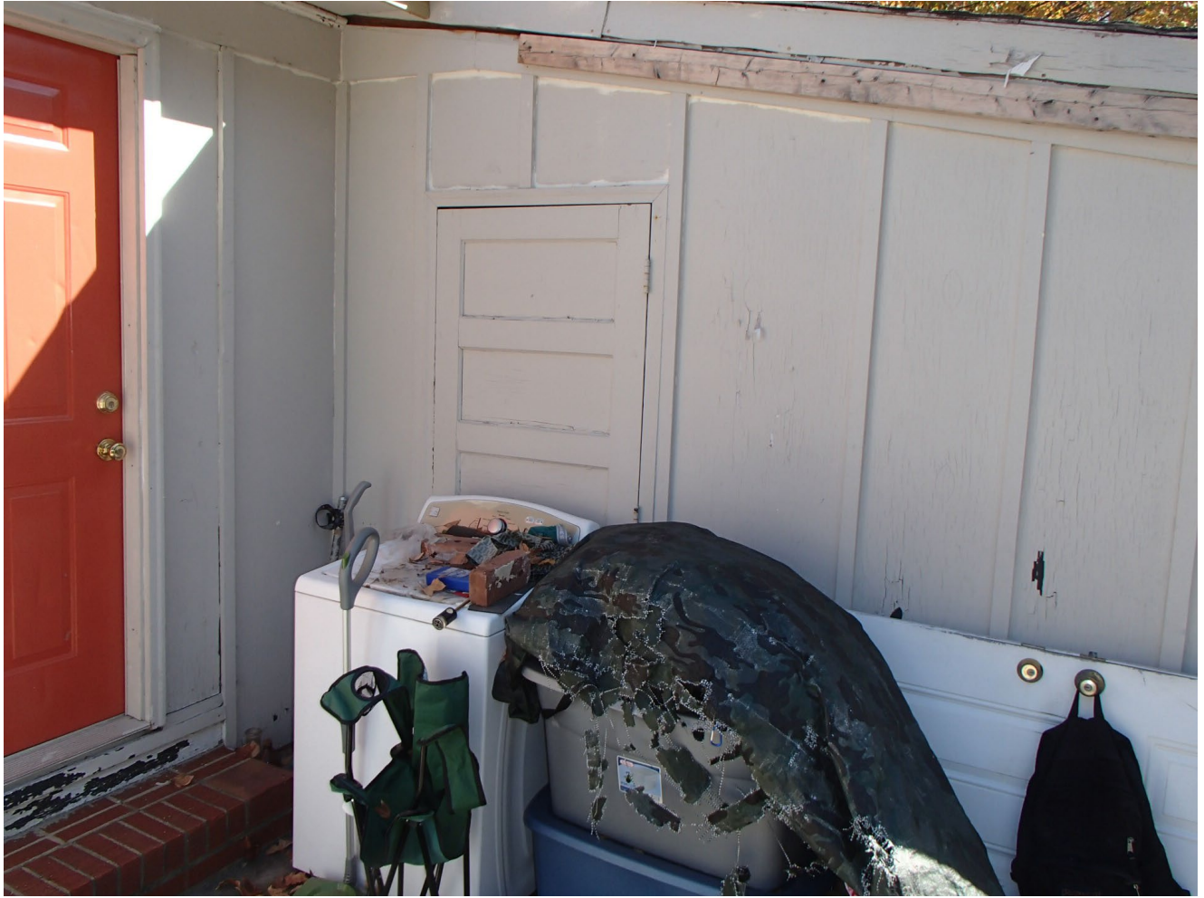
Photo 6 – Side C Wall (left), Side D Wall (right) and Closet Door D1 (right door)
