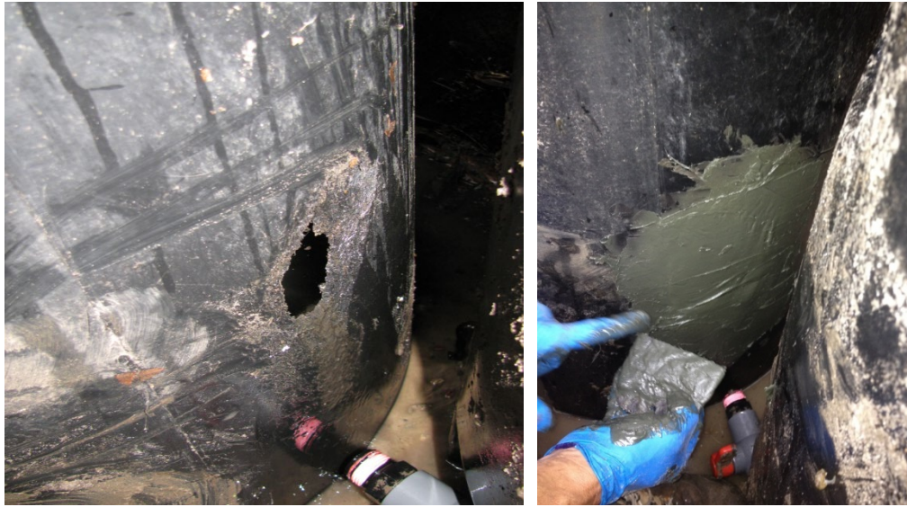
Figure 16. Example of animal damage to cistern and patching of hole. (NCSU BAE)
