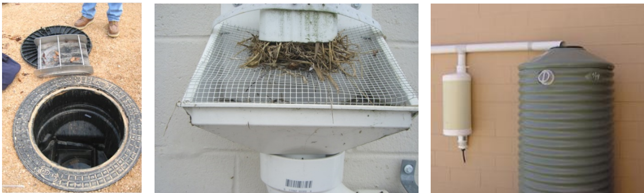
Figure 2. Fine filter used upstream of an underground cistern (left), gutter screen (center), downspout screen (right) (NCSU BAE left and center and UNC-CH right).
