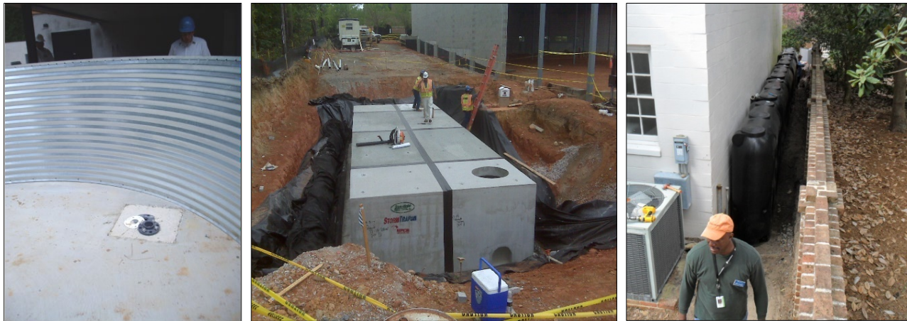
Figure 3. Metal cistern under construction (left), underground concrete vault wrapped in an impermeable liner (center) and a series of plastic cisterns (right) (UNC-CH left and NCSU BAE center and right)
