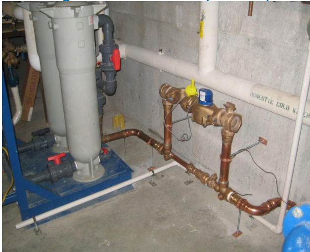
Figure 9. Water Meter (UNC-CH)
