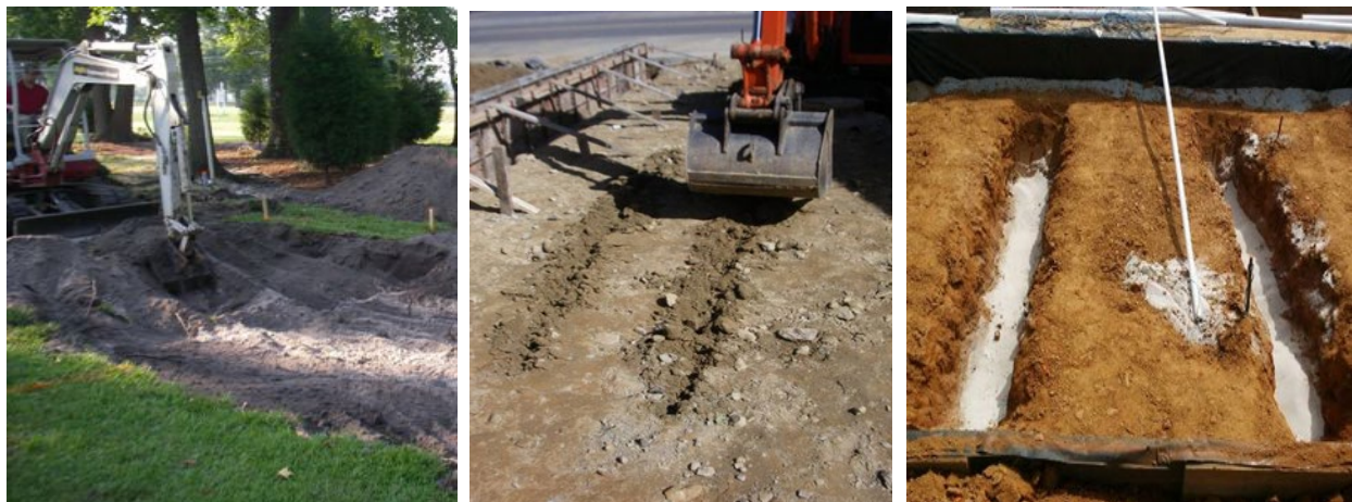
Figure 10. Good Construction Practices, from left to right: Grading from the Side (NCSU), Scarifying the Subgrade (Tyner), Trenching the Subgrade (Tyner)
