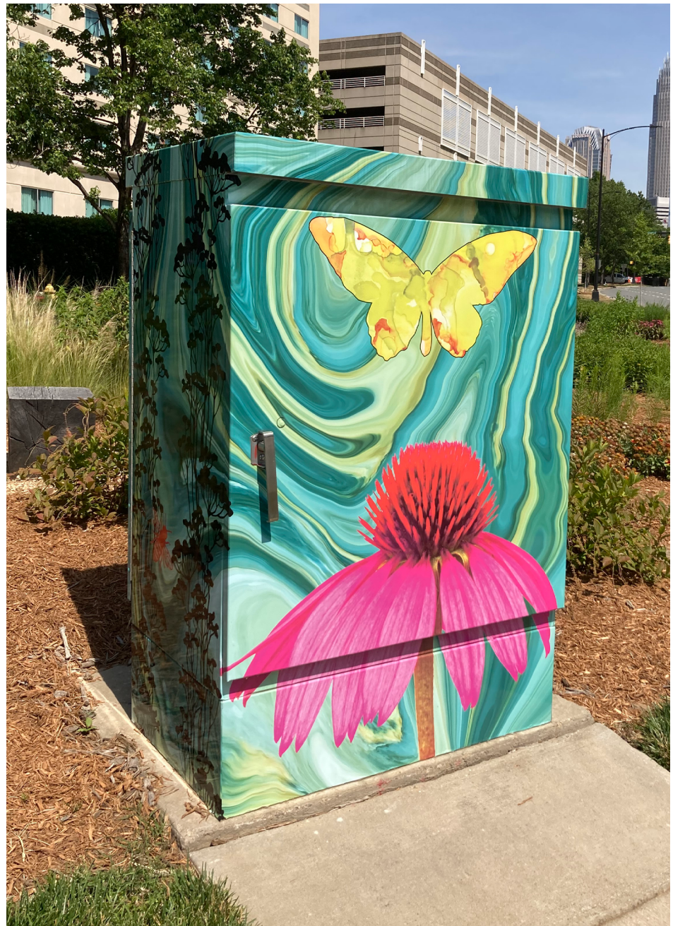
W 4th Street signal cabinet at the Urban Arboretum Trail
