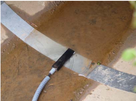
Figure 1: Area velocity meter installed in culvert
