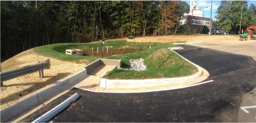
Figure 5: Bioretention area with stormwater inflow monitoring box.
