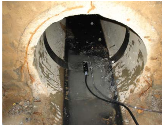
Figure 2: Typical installation of area-velocity probe (left) and sampler intake (right) with expansion bracket
