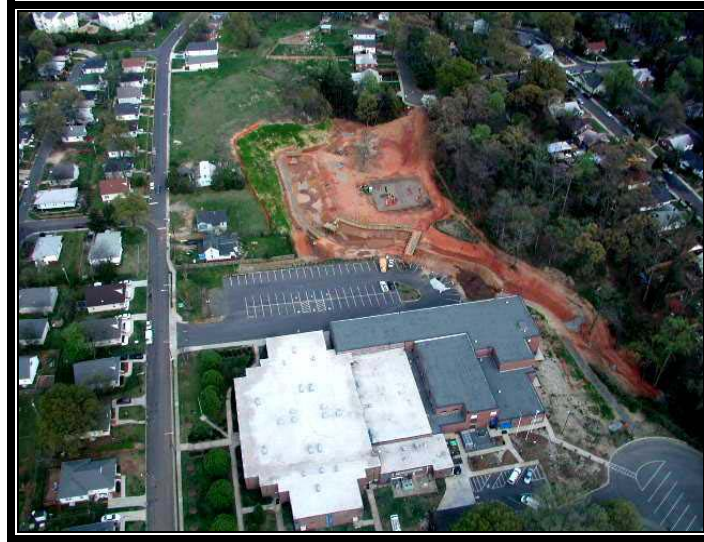
Figure 2. Aerial view of Bruns Ave. School Wetland and contributing watershed during construction
