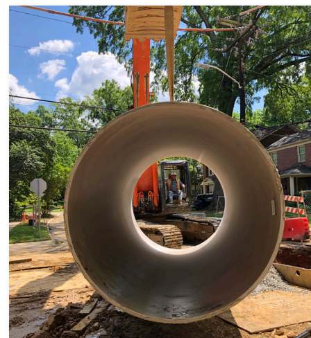
Installation of 84" stormwater pipe at the intersection of Lexington and Oriole Avenues.
