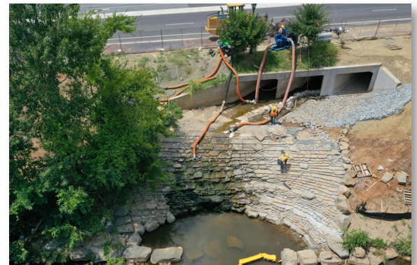
A third box culvert (on the right) was added to the Kenilworth Road box culvert to support the extra flow of stormwater from the Dilworth area.
